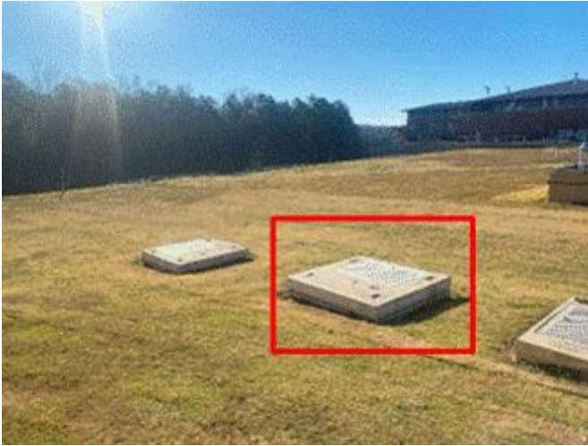
Photo 24 - (SCFP) 96" Valve Operator Vault for RW Equalization Tank Outlet (RW-BFV-11)
