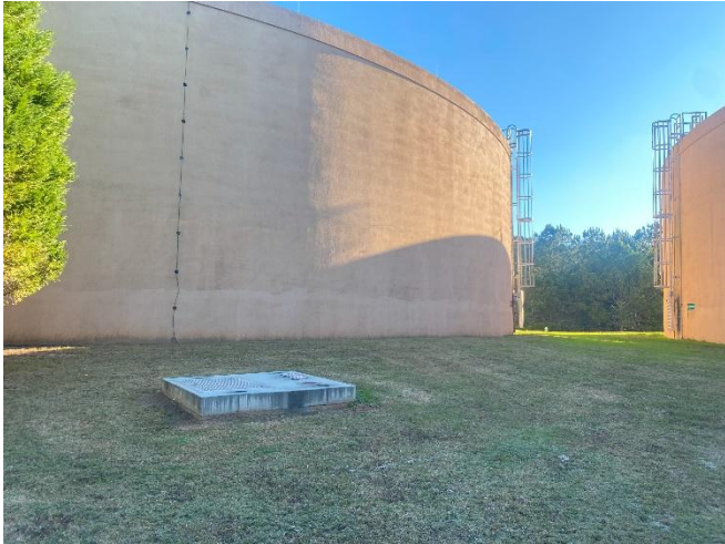
Photo 20 - (SCFP) 54" Valve Operator Vault for RW Equalization Tank No. 1 Inlet (RW-BFV-7)
