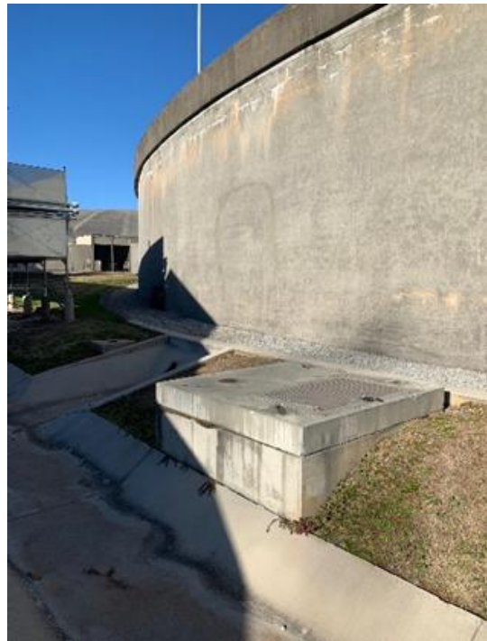
Photo 3 - (LFP) 108" Effluent Valve Operator Vault on Clearwell No. 3
