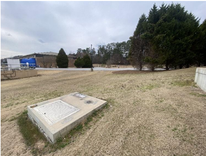
Photo 26 - (SCFP) 54" Valve Operator Vault for RW Equalization Tank No. 1 Outlet (RW-BFV-13)
