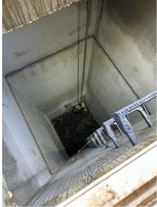
Photo 21 - (SCFP) 54" Valve Operator Vault Interior for RW Equalization Tank No. 1 Inlet (RW-BFV-7)
