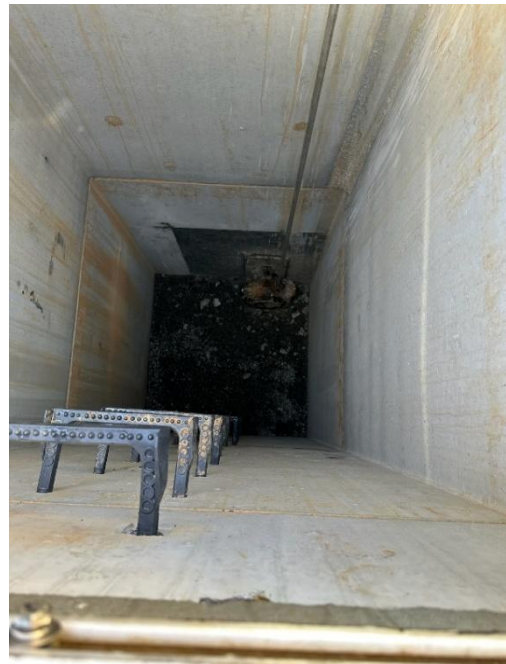
Photo 27 - (SCFP) 54" Valve Operator Vault Interior for RW Equalization Tank No. 1 Outlet (RW-BFV-13)
