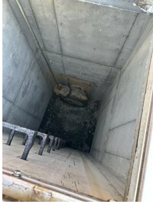
Photo 25 - (SCFP) 96" Valve Operator Vault Interior for RW Equalization Tank Outlet (RW-BFV-11)
