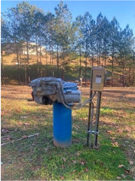
Photo 12 - (SCFP) 72" Electrically Actuated Valve (RW-BFV-1)
