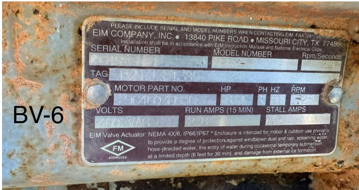
Photo 19 - (SCFP) 72” Motor Operator Nameplate Data (RW-BFV-6)
