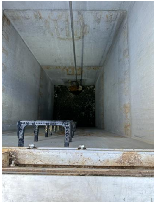
Photo 23 - (SCFP) 54" Valve Operator Vault Interior for RW Equalization Tank No. 2 Inlet (RW-BFV-8)
