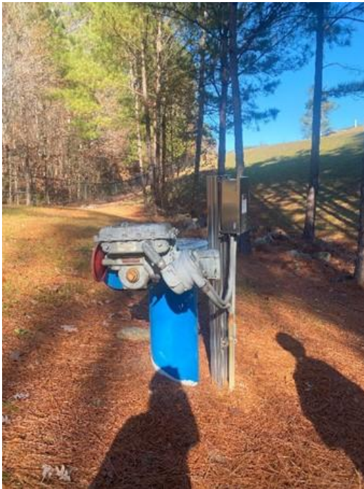
Photo 14 - (SCFP) 72" Electrically Actuated Valve (RW-BFV-5, RW Supply Valve - West)
