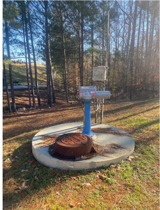
Photo 13 - (SCFP) 72" Electrically Actuated Valve (RW-BFV-4)
