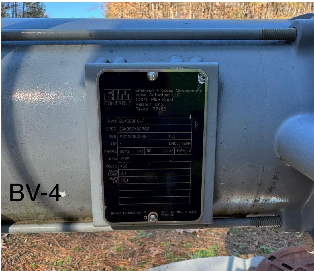
Photo 17 - (SCFP) 72” Motor Operator Nameplate Data (RW-BFV-4)
