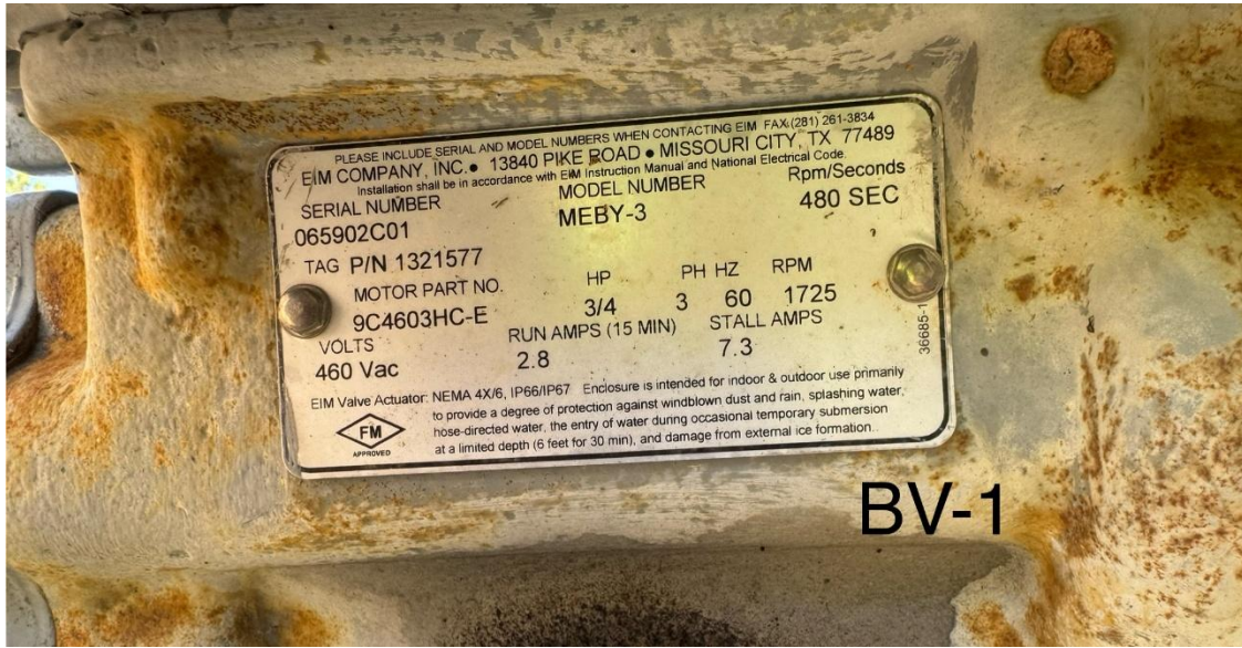
Photo 16 – (SCFP) 72” Motor Operator Nameplate Data (RW-BFV-1)
