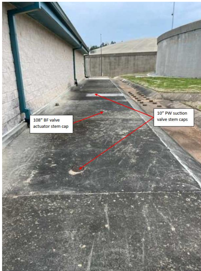
Photo 6 – (LFP) HSPS 108" Valve Actuator Location
