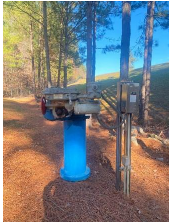
Photo 15 - (SCFP) 72" Electrically Actuated Valve (RW-BFV-6, RW Supply Valve - East)
