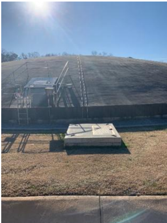
Photo 2 - (LFP) 108" Influent Valve Operator Vault Clearwell No. 3
