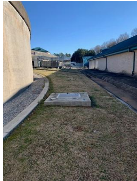
Photo 5 - (LFP) 108" Effluent Valve Operator Vault on Clearwell No. 4
